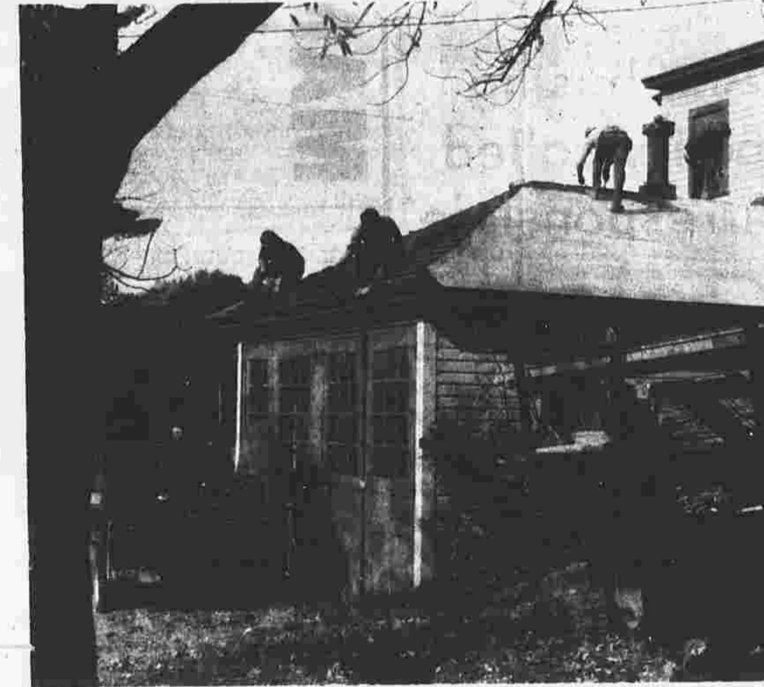
Workers from M. Dzan Roofing Contractors of South Windsor replace shingles on the roof of equipment room of the town fire museum at the corner of Hartford Road and Pine Street.
